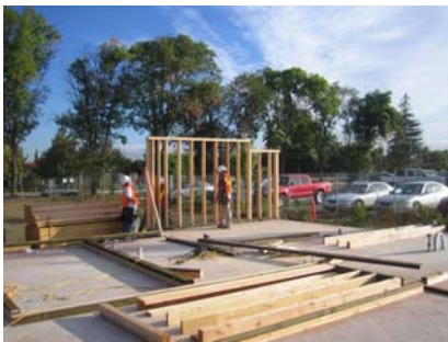
October 4 th . 8:30am. Our devoted Project Superintendent and friend Tim Thompson sends us the picture of another milestone: JW House's very first wall is going up! In no time, the "entire world" will be excited about what is happening 😊!
